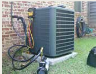
Pre-season HVAC tune ups
