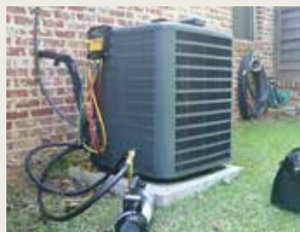
Pre-season HVAC tune ups
